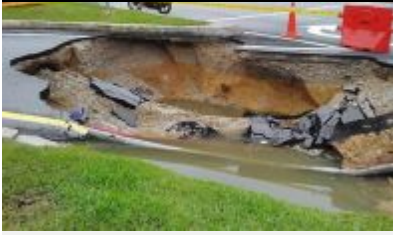
Growing sinkhole forces road closure in Bandar Utama
